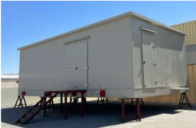
33/11 KV PRIMARY PACKAGE UNIT
