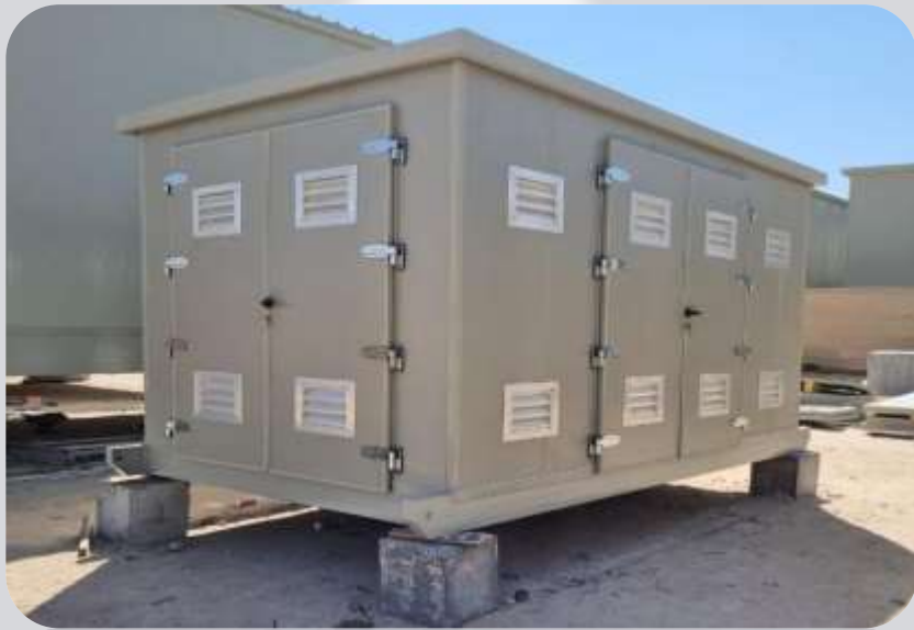
11 KV GRP PACKAGE UNIT
