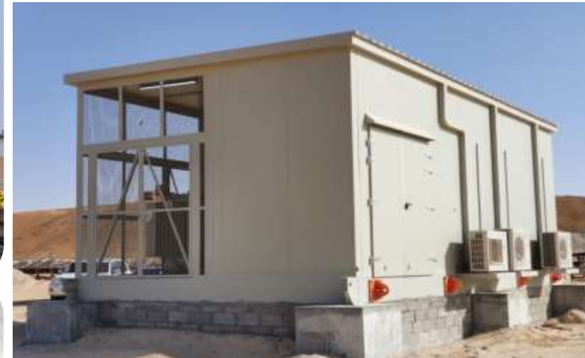
22 KV GRP PACKAGE UNIT
